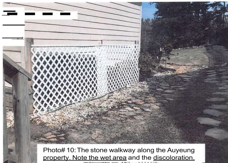
Photo# 9: Photo shows the stone walkway. Note the area and the discoloration.
