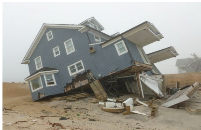
Figure 13: House in Mantoloking Knocked Off Foundation by Superstorm Sandy Storm Surge 284
