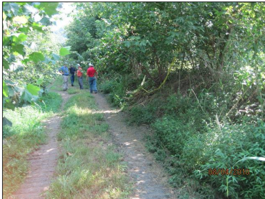
3-2 BEHIND WEST DIKE LOOKING NORTHWEST. VEGETATION AND TREES ON WEST DIKE (ON RIGHT SIDE OF PHOTO)
